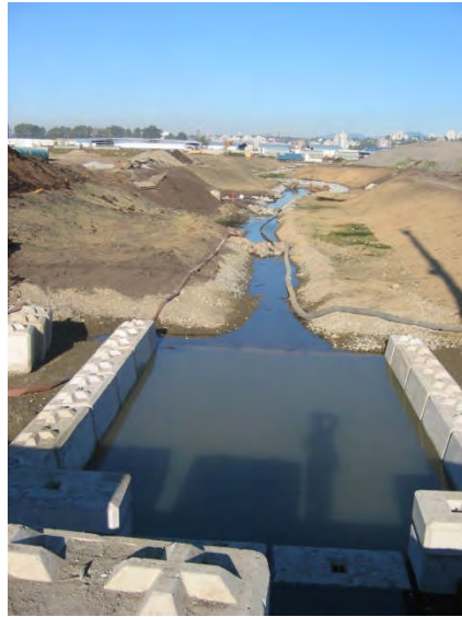
Figure 8: Example of Sediment Trap (Scott Creek in Surrey, BC)
